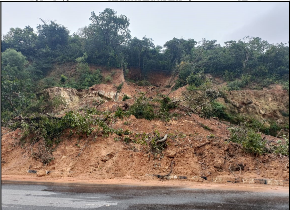
Fig. 2.2: Deep rotational failure with possible piping at chainage 160.080
