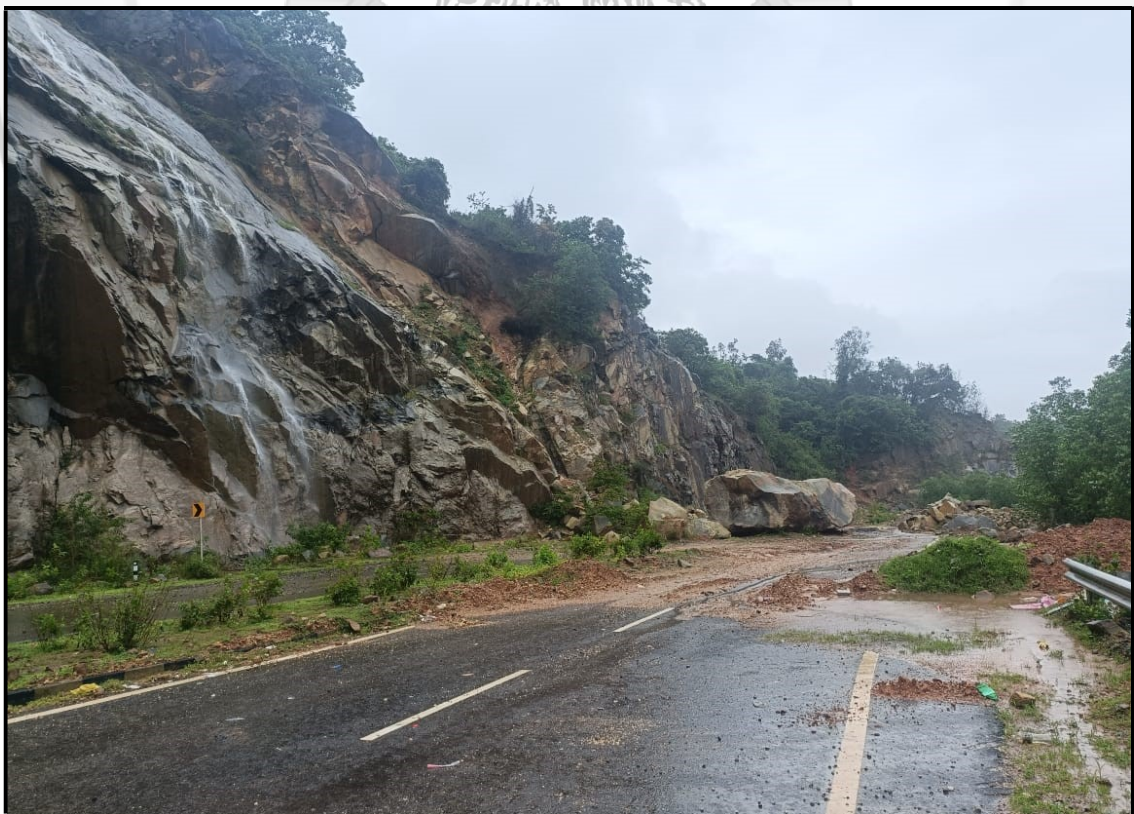
Fig. 2.3: Rockfall incidence at chainage 111.400
