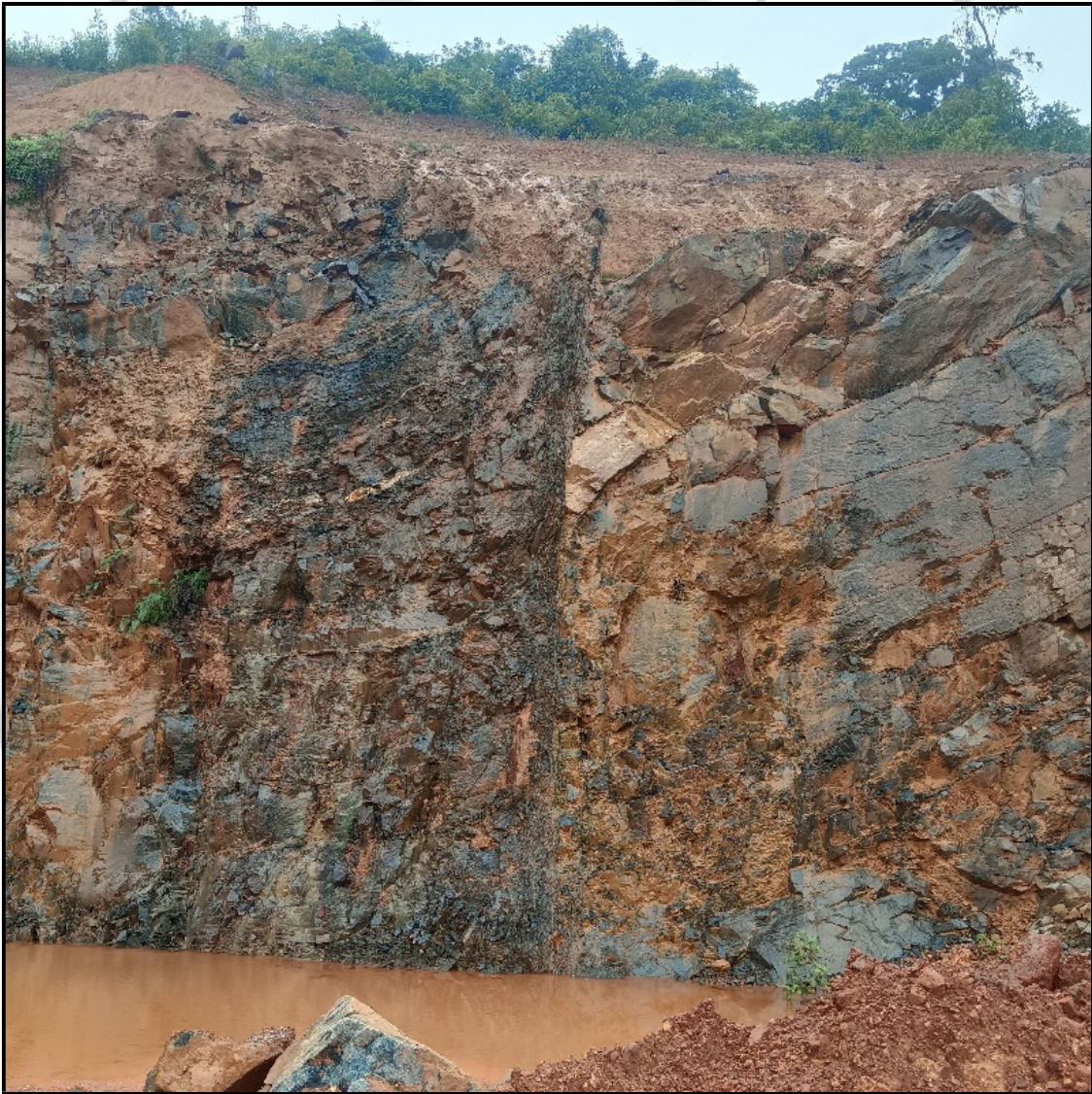
Fig. 1.5: Minor Fault observed at the base of the cut slope on the right flank of the slide
