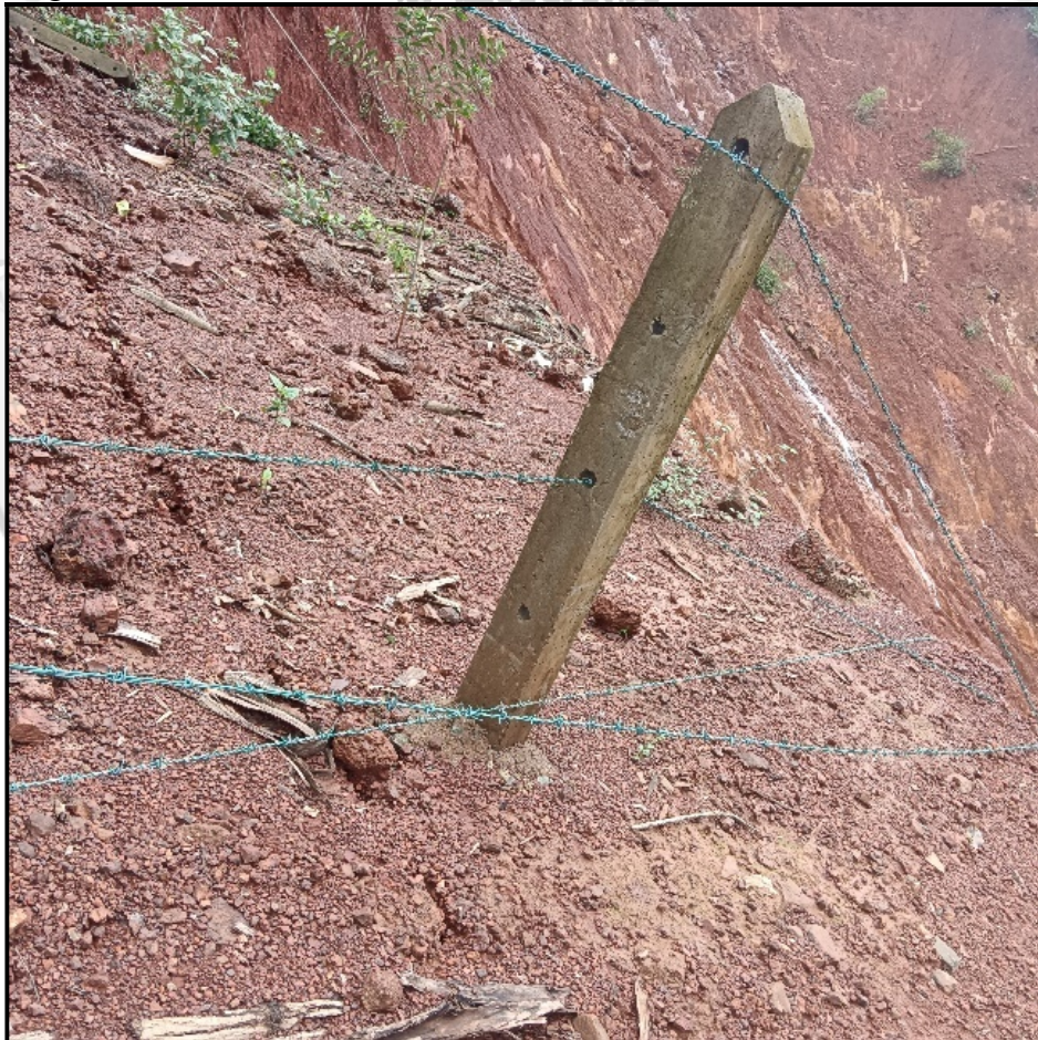
Fig. 1.12: Transverse cracks at the right flank of the landslide trending N15°
